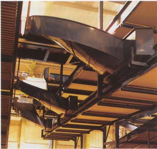
1 CHUTES FEEDING BELT CONVEYOR
